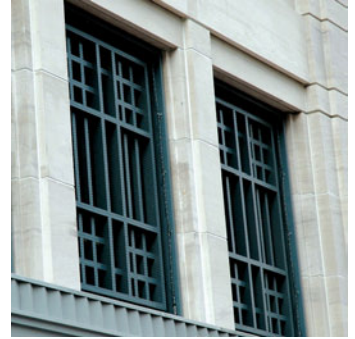
Exterior air intake grilles
